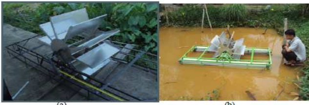
Figure 3: (a) The wheel and supporting frame in construction. (b) The floating test is conducted with PVC pipes at the left and right sides.
